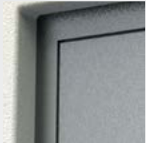
Flush alignment on the inside
